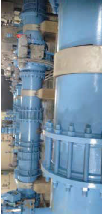
Piping for water plant pumps
