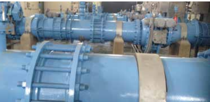
Piping for water plant pumps
