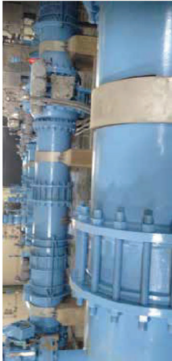
Piping for water plant pumps
